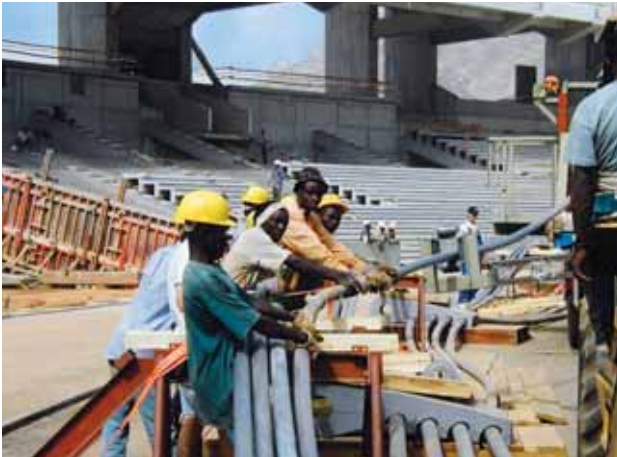
Installation of the ring cable connector is always carried out manually – here inserting and aligning of connectors, National Stadium Main Bowl Complex, Abuja.
