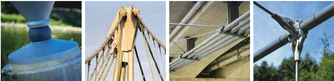
Construction elements that require special attention: i.e. pylon foot, pylon head, cable clamps, hanger cable clamps. (left to right).
