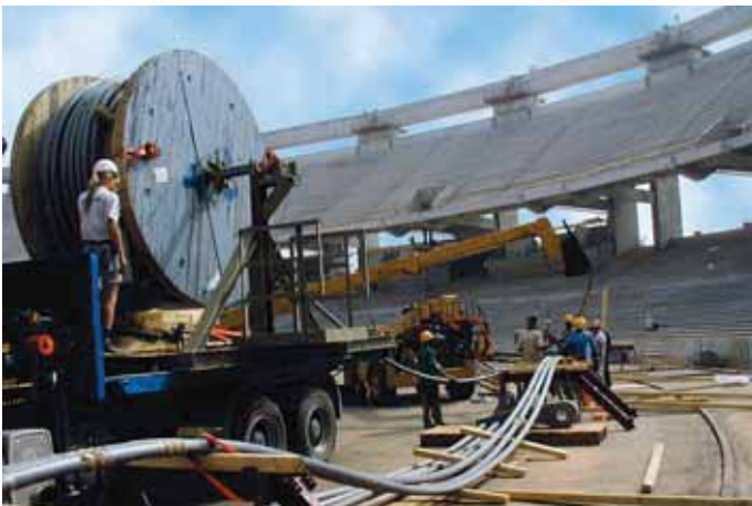
Laying out VVS-cables with a mobile unreel stand – here a tensioning ring, National Stadium Main Bowl Complex, Abuja.
